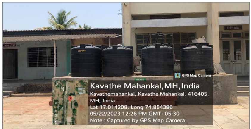
Rain water harvesting facility in the premises
